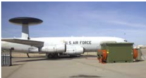
Piller equipment at AWACS bases worldwide.
