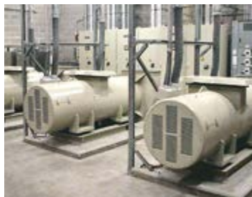
Central system with Piller Motor-Generator Sets.
