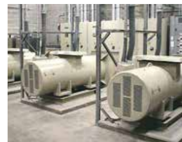
Central system with Piller Motor-Generator Sets.
